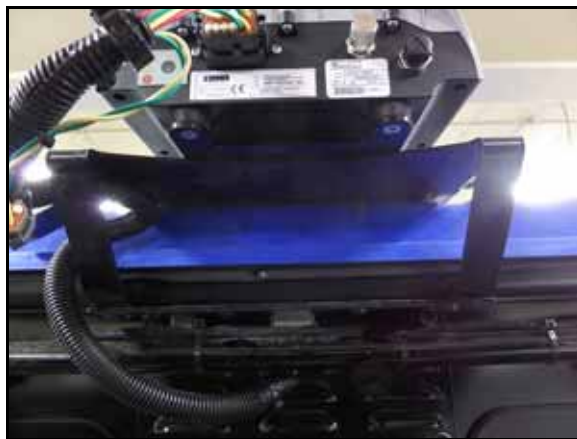
FIGURE 8. RS1 Harness Connected to Bulkhead
