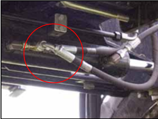
FIGURE 8. Installed Left Steering Hose on Right Steering Cylinder
