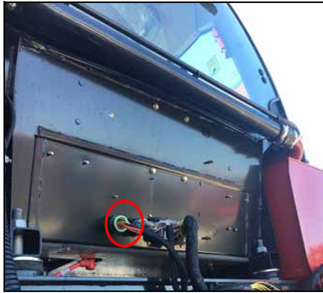
FIGURE 20. RS1 Tee Cable Connected to Machine's Bulkhead
