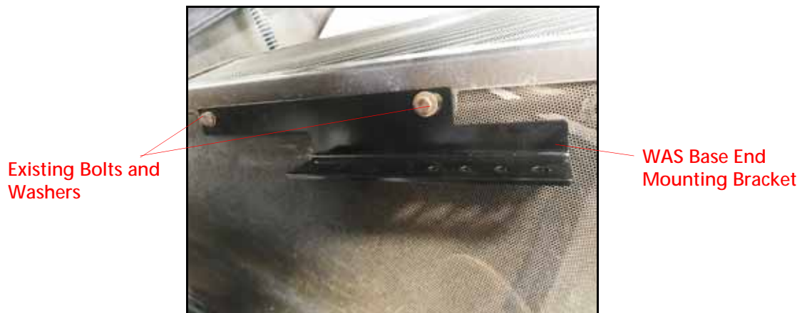
FIGURE 4. 3XXX WAS Bracket on Installed on the Radiator Cover
