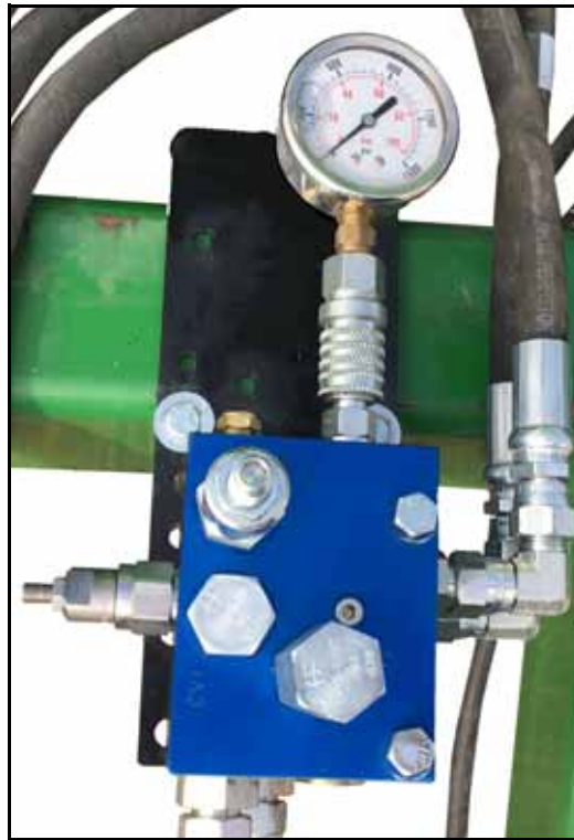
FIGURE 3. Installed Hydraulic Pressure Gauge
