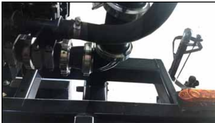
FIGURE 11. Flowmeter Connected to Elbow
