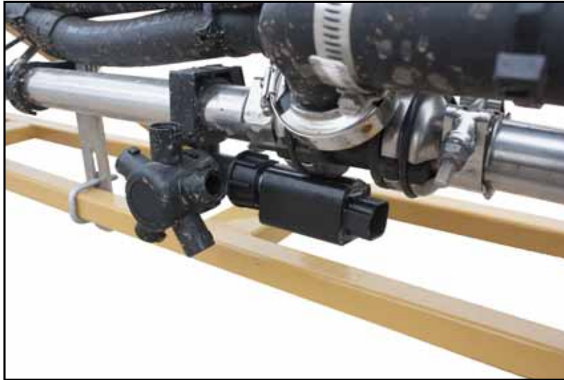
FIGURE 10. Modified Nozzle Control Valve Installation
