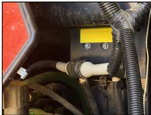
FIGURE 3. 15' RS1 Tee Cable Connected to Machine's Power Cable
