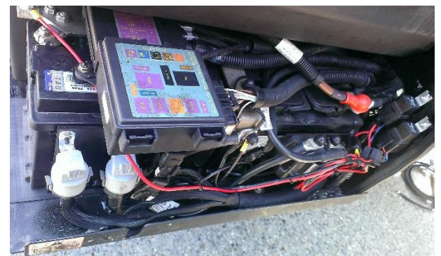
Figure 3 mounted relays and fuses.
