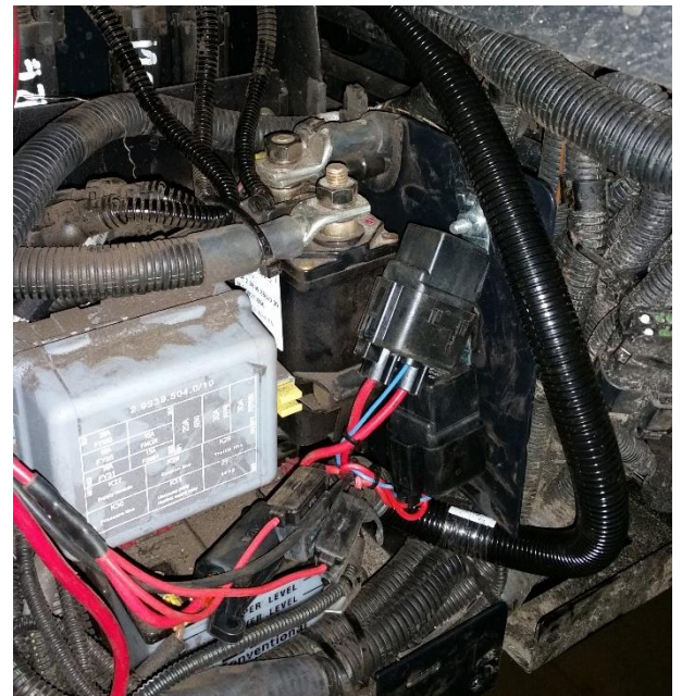
Figure 3 Mounted relays and fuses.
