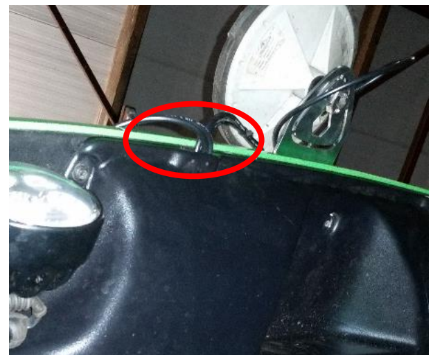
Figure 10 Location where antenna cables can be lead into the cabin.
