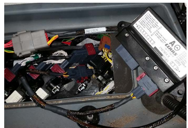
Figure 5 Cabling connected to the Claas ATP2 module and SBG Claas ATP Ready harness.
