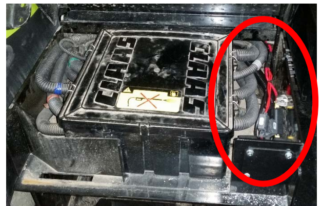
Figure 2 Correctly mounted relays and fuses.
